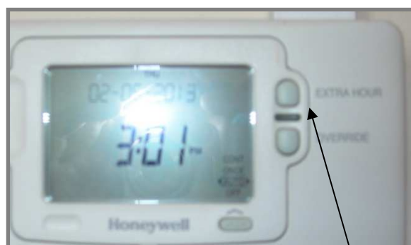
Photo of a heating programmer with an 'extra hour' button taken at Eynsham Baptist Church.
