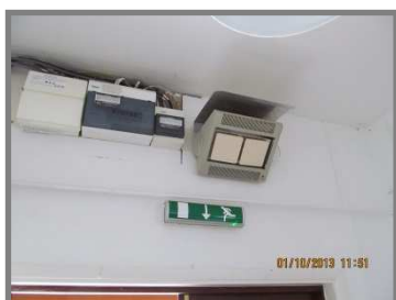
Existing 2kW Electric Radiant Heater
